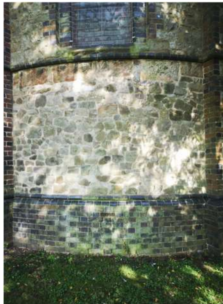
Image 4 – Diagonal crack in the rear elevation
