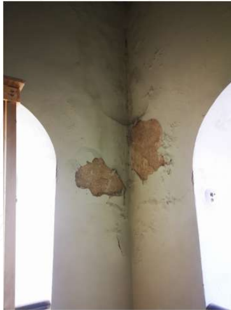
Image 20 Flaked lime plaster at mezzanine landing level
