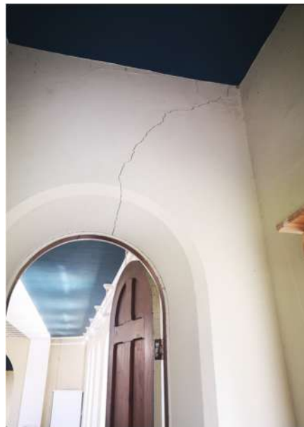
Image 21 Diagonal cracks above door opening at mezzanine floor level
