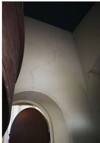
Image 18.4 Diagonal cracks above the door opening between the south bay and the Nave
