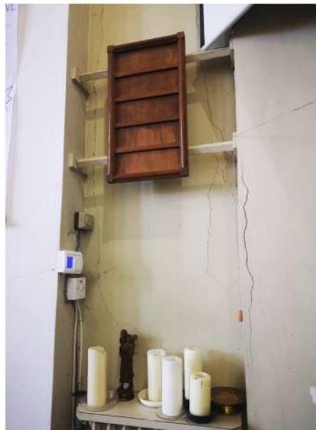
Image 15.3 Vertical cracks and flaked plaster in the rear wall
