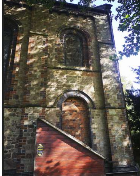
Image 1 – Helifix crack repairs carried out in the past
