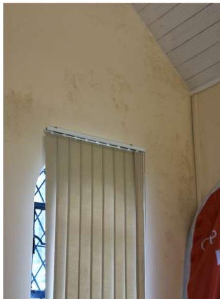
Image 24 Dampness in the East side wall of Library
