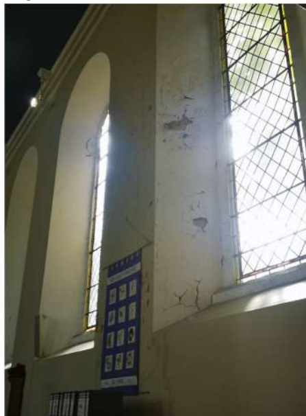
Image 13 – Multiple cracks and flaked plaster work in south elevation window
