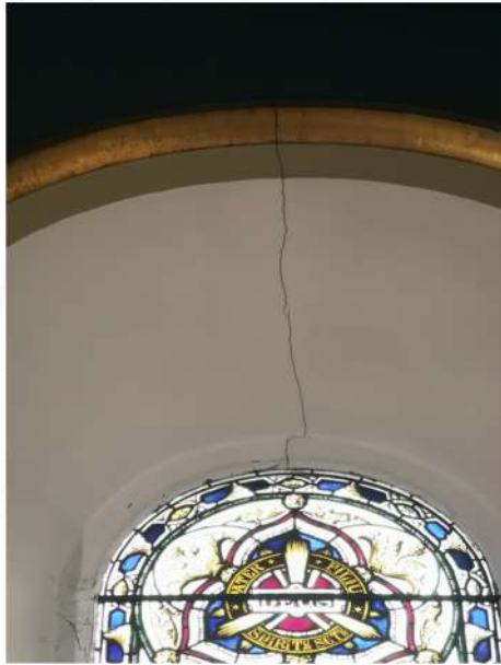
Image 17.2 Vertical crack above window within Apse
