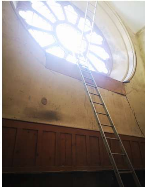
Image 22.1 Diagonal cracks below the Large wheel window opening
