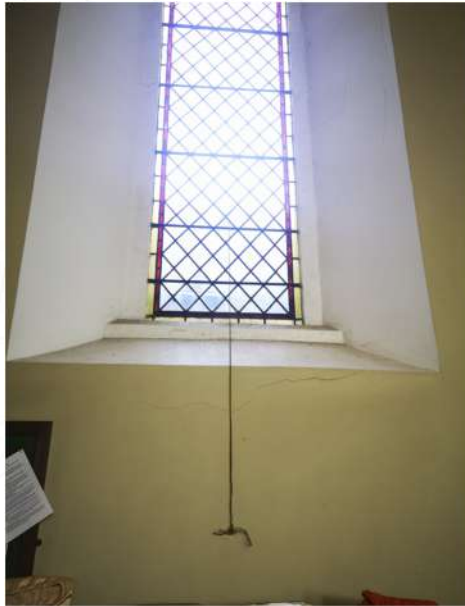
Image 11.1 – Multiple hairline cracks around the window
