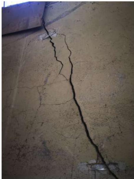
Image 22.2 Diagonal cracks below the Large wheel window opening
