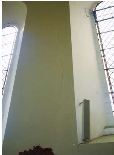
Image 12 – Vertical cracks between windows
