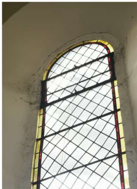
Image 11.6 – Multiple hairline cracks around the window
