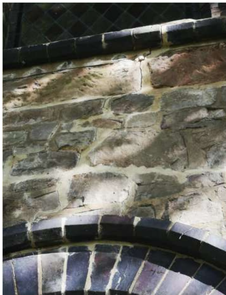
Image 2 – Diagonal cracks above window -within the helifix repair
