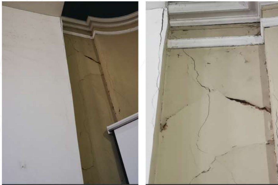
Image 15.2 Vertical cracks and flaked plaster south east corner wall
