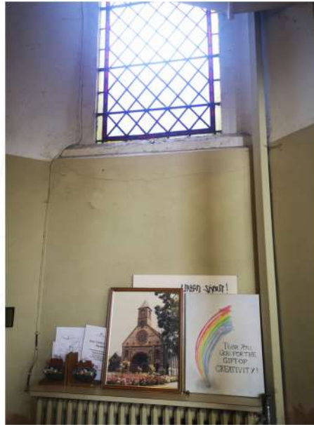
Image 9– Horizontal cracks below the front elevation window sill level
