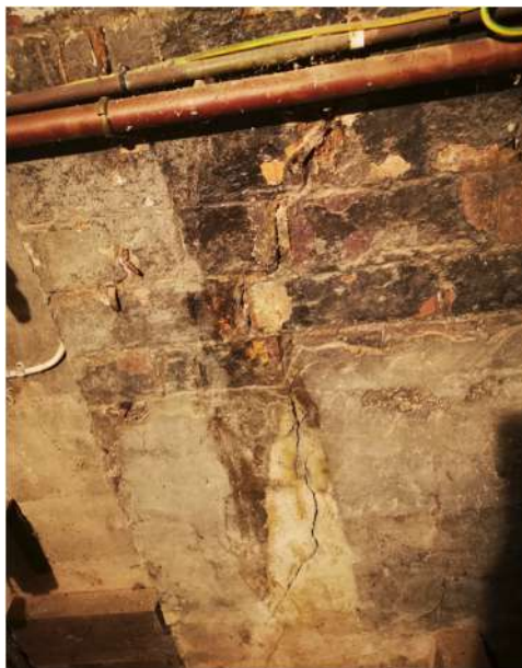
Image 7.1 – Cracked basement – East side wall
