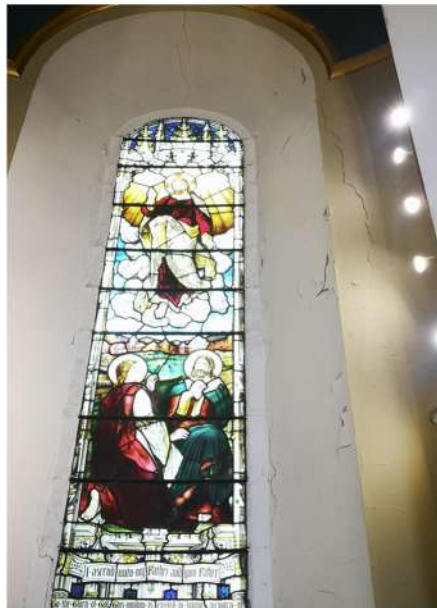
Image 17.3 Multiple cracks around the window opening in Apse
