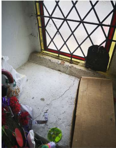
Image 19.1 Cracks around the front elevation window within the staircase room
