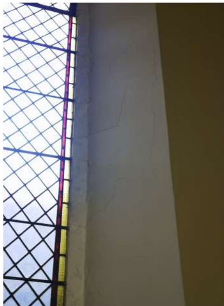
Image 11.2 – Multiple hairline cracks around the window
