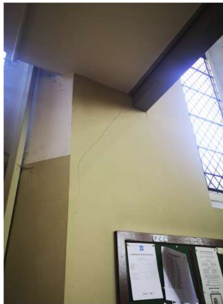
Image 10– Diagonal cracks below the timber beam at mezzanine level
