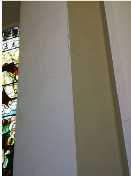
Image 14 – Vertical cracks in the south side pier between Apse and Nave
