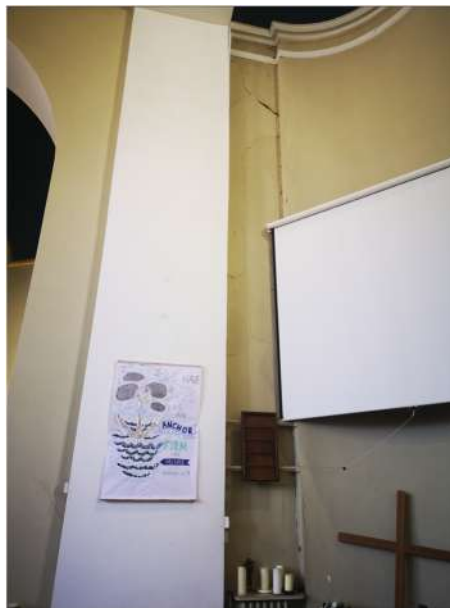
Image 15.1 – Vertical cracks and flaked plaster in the rear wall
