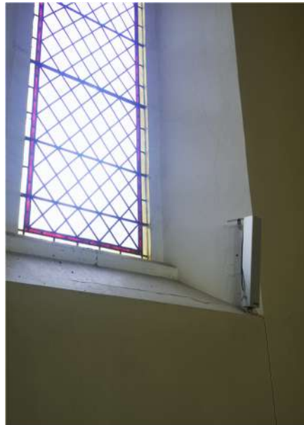
Image 11.4 – Multiple hairline cracks around the window
