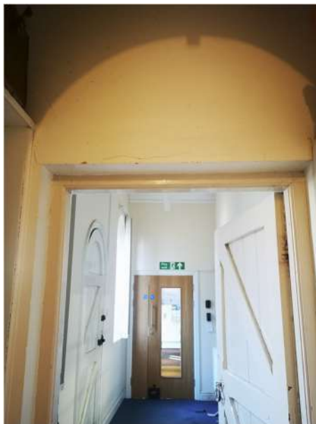
Image 8 – Horizontal cracks above the door opening
