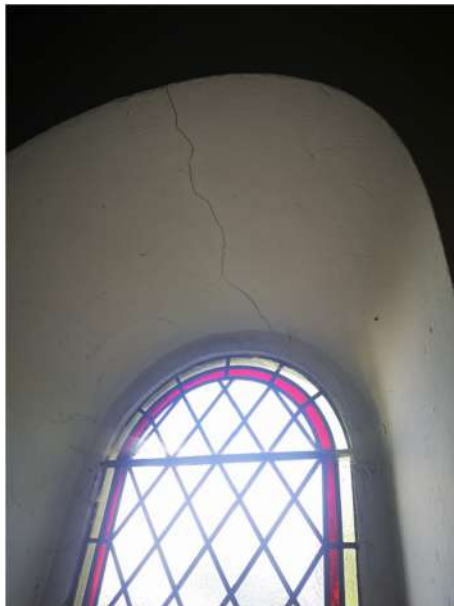
Image 19.2 Cracks around the front elevation window within the staircase room
