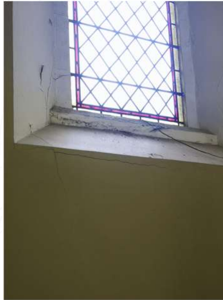
Image 11.3 – Multiple hairline cracks around the window
