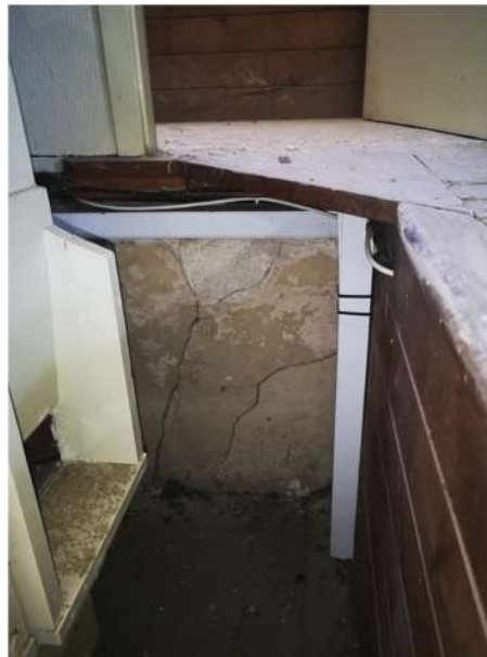
Image 23.1 Diagonal cracks at mezzanine level
