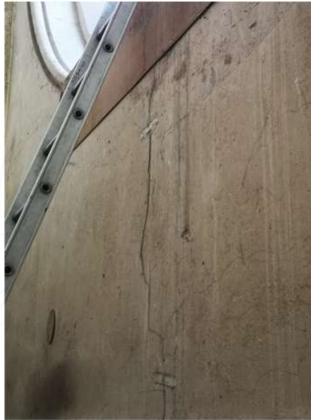
Image 22.3 Diagonal cracks below the Large wheel window opening
