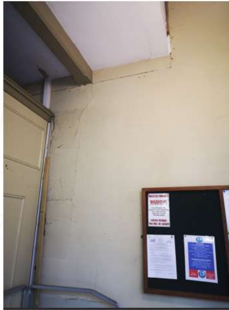
Image 23.2 Diagonal cracks at mezzanine level extended below
