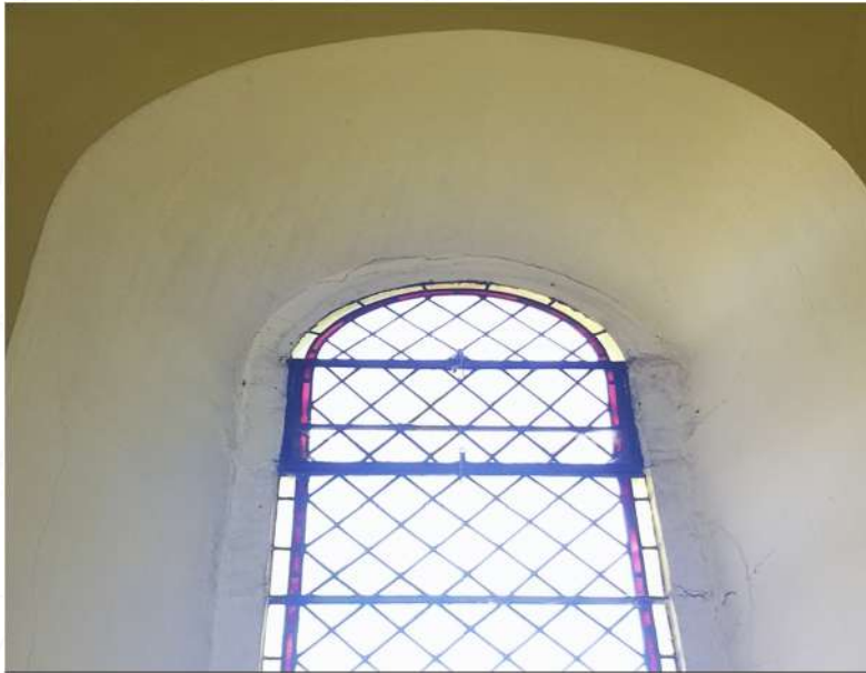
Image 11.5 – Multiple hairline cracks around the window
