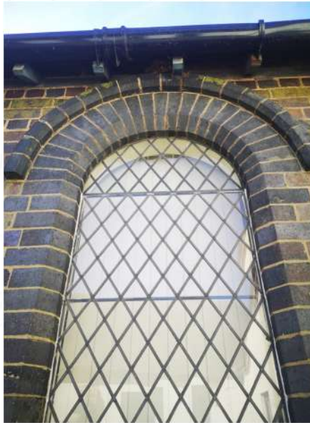
Image 5 – Cracked joint at brick lintel to the side elevation
