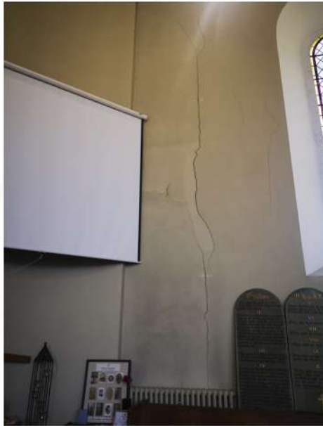
Image 16 Full height vertical cracks in the South east corner of south elevation wall
